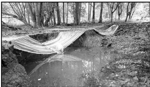
Some of the damage caused by the flooding.
